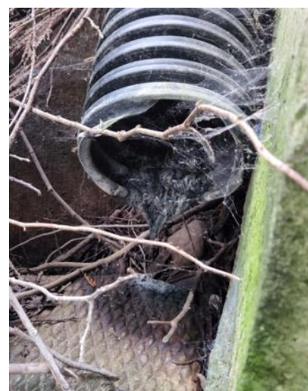
Potential illegal "straight pipe" in an old residential area that is suspected of releasing wastewater from a malfunctioning septic system to a nearby stream.
