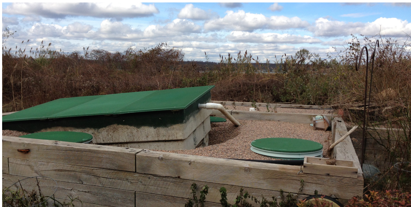
Figure 10: Flood-damaged advanced nitrogen reducing OWTS in coastal Rhode Island. Storm surge flooding displaced buoyant components of the OWTS. This type of damage can be mitigated with proper anchoring.
